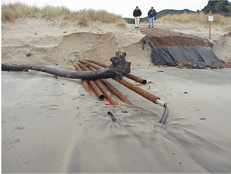
Figure 2-1. Cable landing infrastructure exposed by coastal erosion in the Rockaway Beach, Oregon area in late 2001. Image source: J. Allan.
